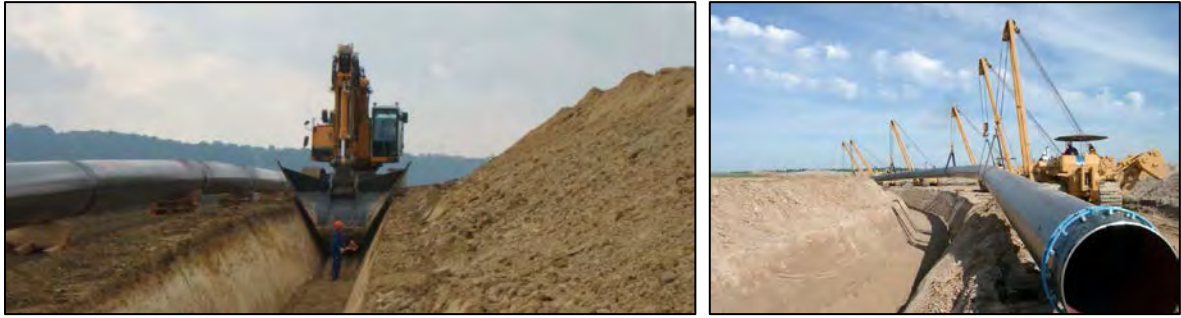
Figure 6-21 Onshore pipeline trench excavation (left) and the pipeline being lowered into the trench.
