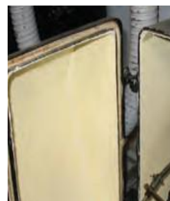
Seal of 11kV oil circuit breaker (OCB) closing contactor box
