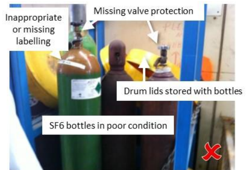
SF6 cylinders with missing valve protection and inadequate labelling
