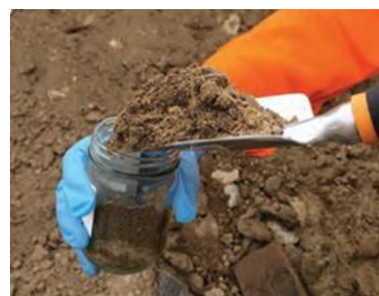
Spoil from below the slab should be assumed SCW unless tested otherwise
