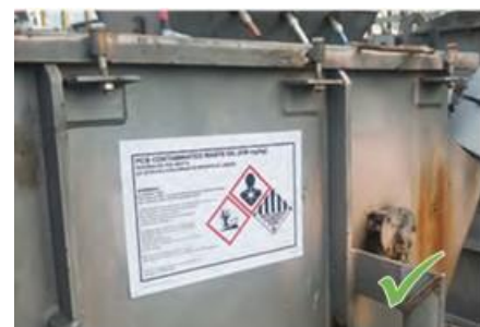
PCB waste labelled ready for collection
