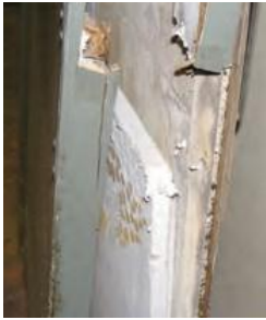
Damaged fire door exposing asbestos core
