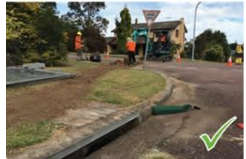
Controls used to protect stormwater inlets
