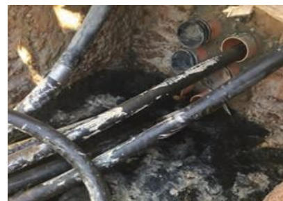
Unknown material seeping into trench will need to be assessed
