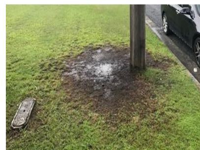
Contamination from a leaking pole transformer
