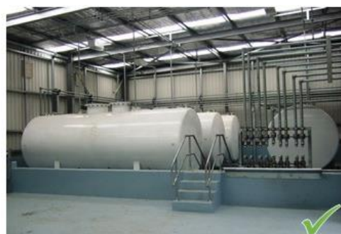
Permanent storage facilities should always be the first preference
