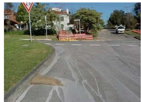
Saw-cutting slurry has not been contained effectively
