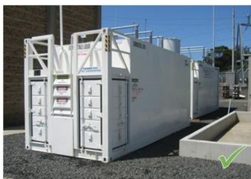
Self-bunded (double-walled) transportable tanks can be used for permanent storage
