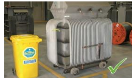
Spill kits should be readily available near oil storage areas
