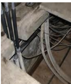
Feeder cables at zone substation
