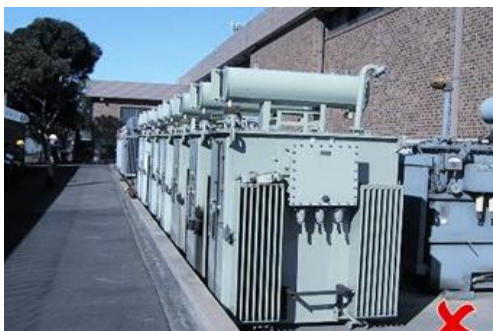
Equipment stored too close to the bund wall means leaks may not be contained
