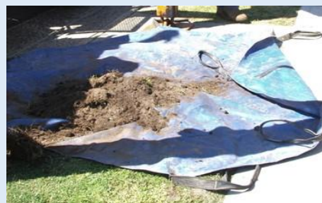
Spoil temporarily placed on tarp to prevent run off and assist clean up
