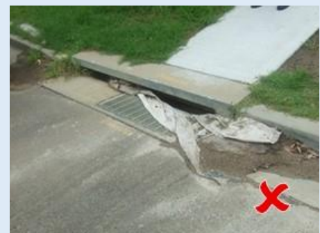
Regularly inspect and maintain sediment controls
