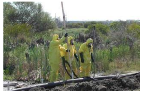
Working in contaminated areas may require special PPE
