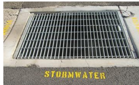
Check whether nearby drains go to stormwater, sewer or the oil containment tank
