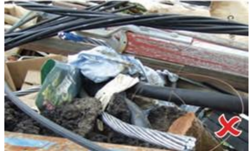
Example of poor waste segregation
