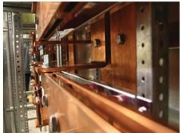
Low voltage busbars
