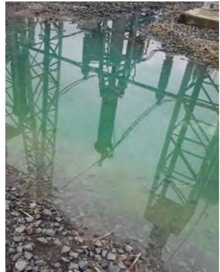
Unusually coloured water is an indicator of contamination
