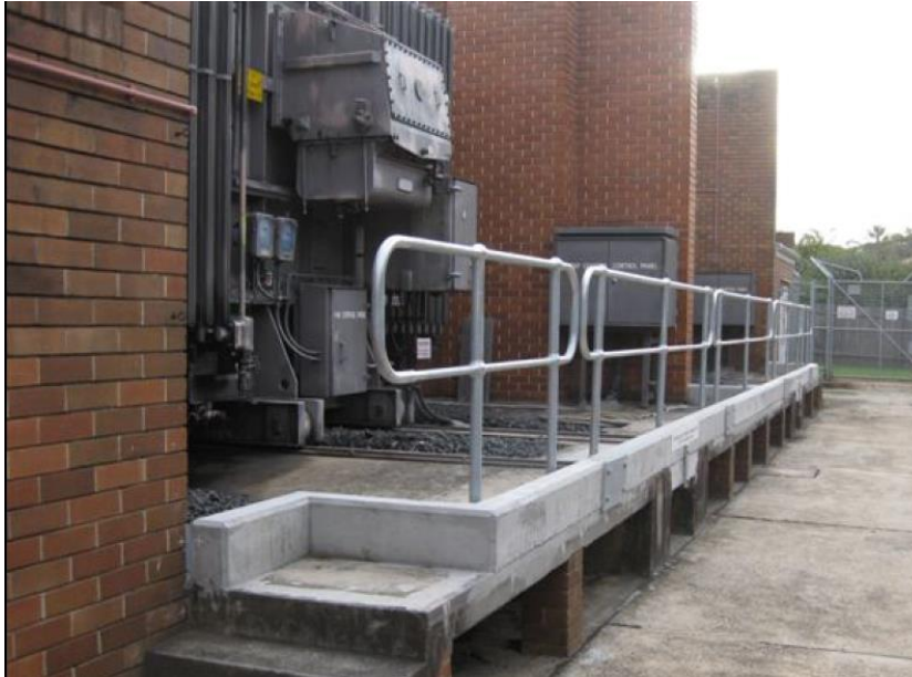
Figure 2: Oil Containment Bund with Gravel
