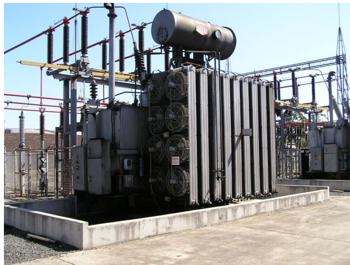
Figure 1: Typical Oil Containment Bund
