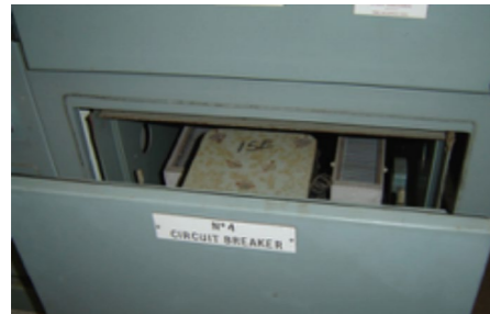
ACM asbestos arc shields
