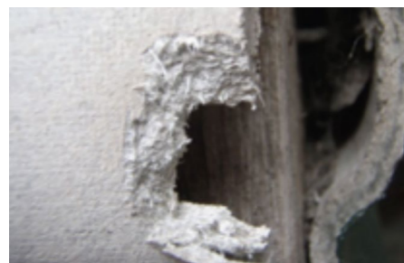
ACM old water pipe
