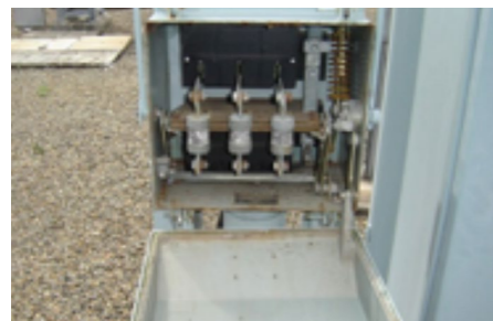
ACM rope seals of fuse box
