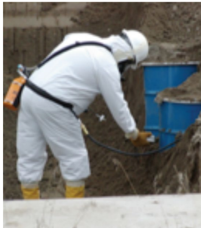
Contamination may require special PPE for the safety of workers
