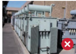
Equipment stored too close to bund wall.
