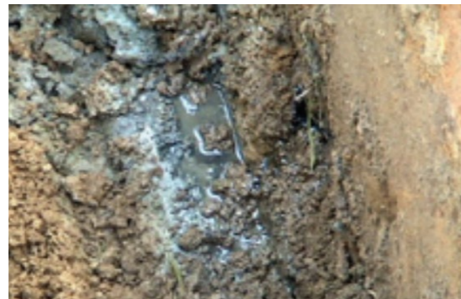
Excavation reveals oil contamination in an excavation next to a Transformer Bund
